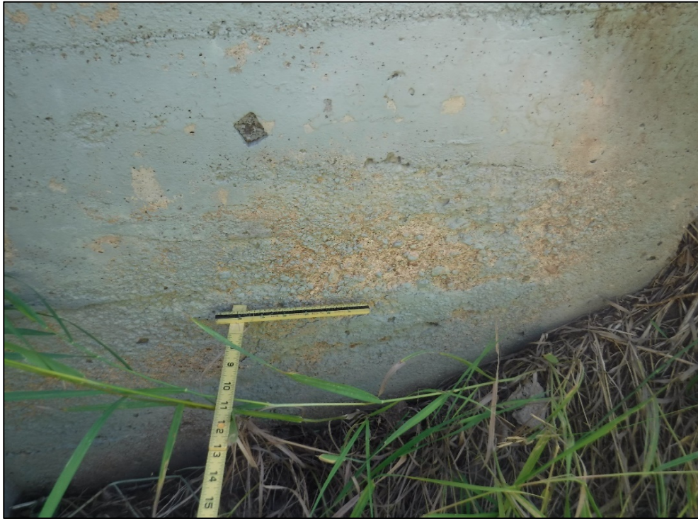
Northeast wingwall has S2 scaling.
