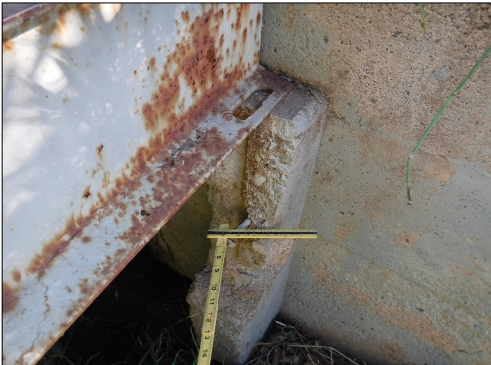
Abutment 14 east end spall with bearing area loss and missing connection.
