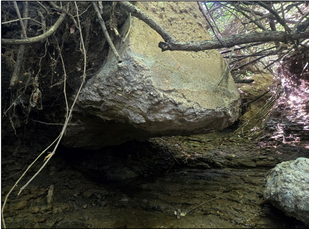
Pier 6 west footing undermined.
