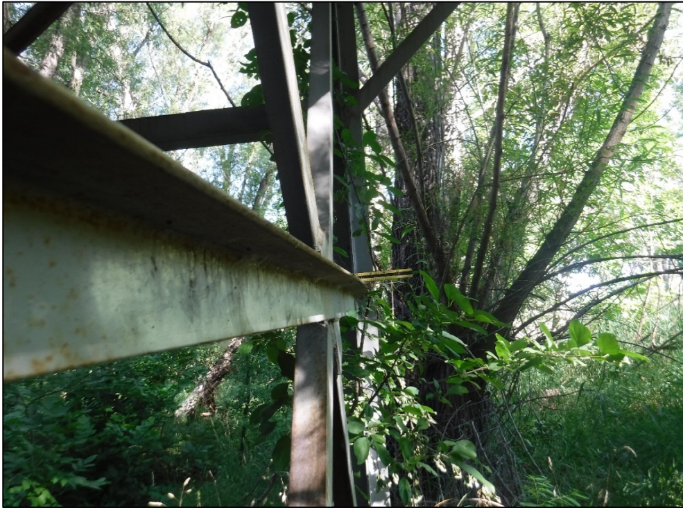
Pier 7 trestle middle horizontal member bent north.
