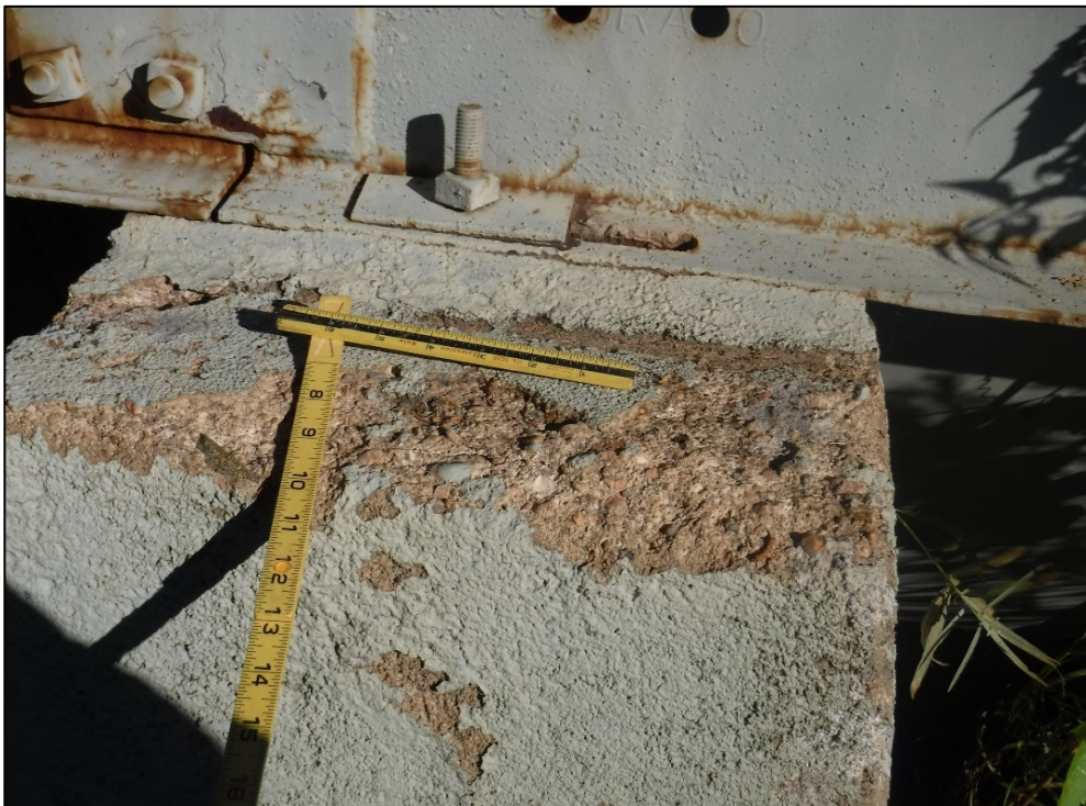
Pier 13 east column at top has S2 scaling.
