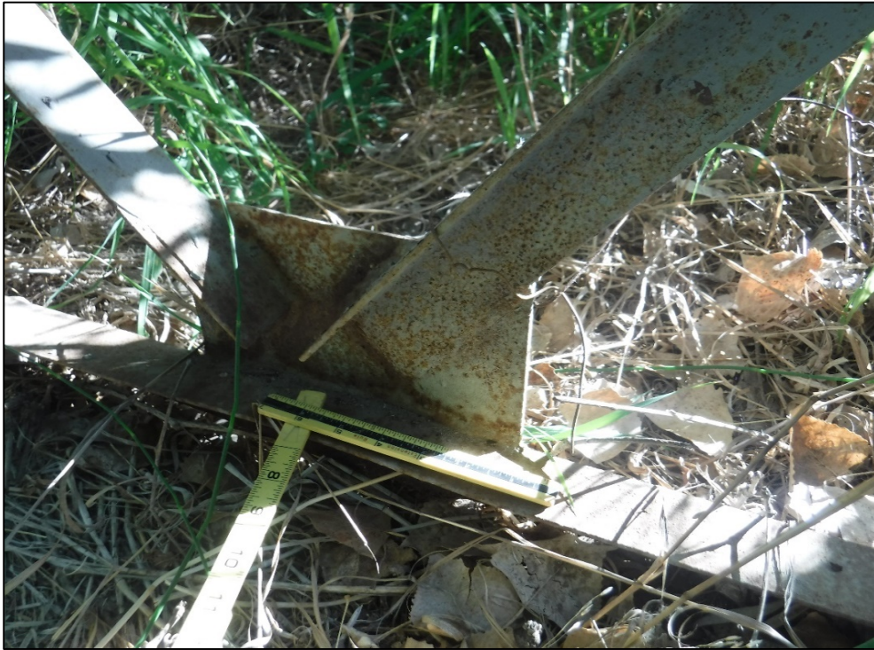
Trestle diagonals have spotty R1 corrosion, typical.
