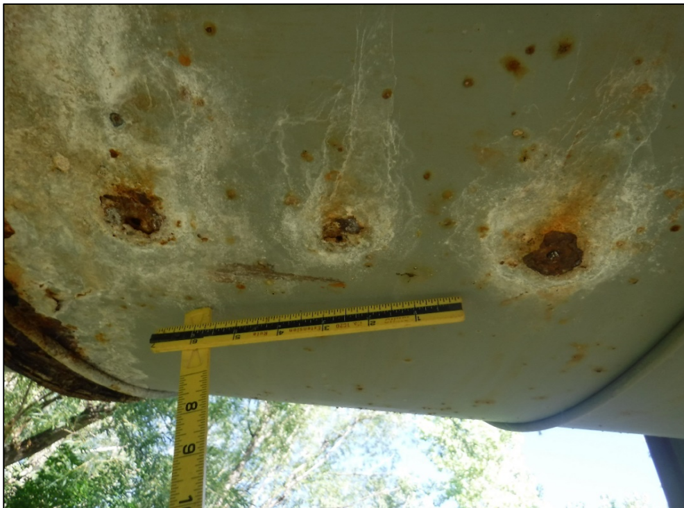
Deck underside in Span 8 has area of pinhole corrosion.
