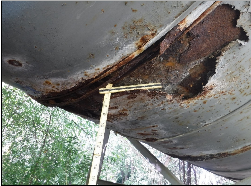
Deck underside in Span 11 has area of R4 corrosion.
