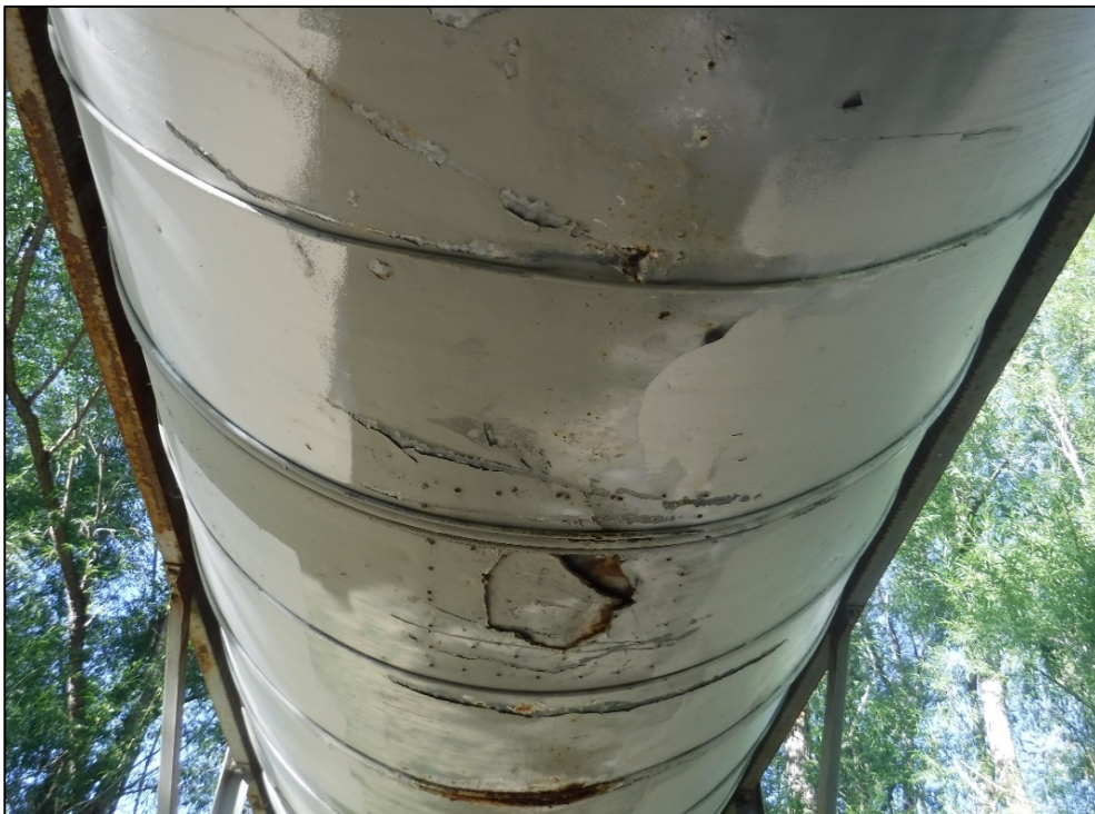
Deck underside in Span 9, 6 feet x 3 feet area of impact damage.
