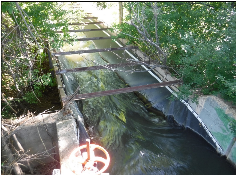
Flume looking north (topside).
