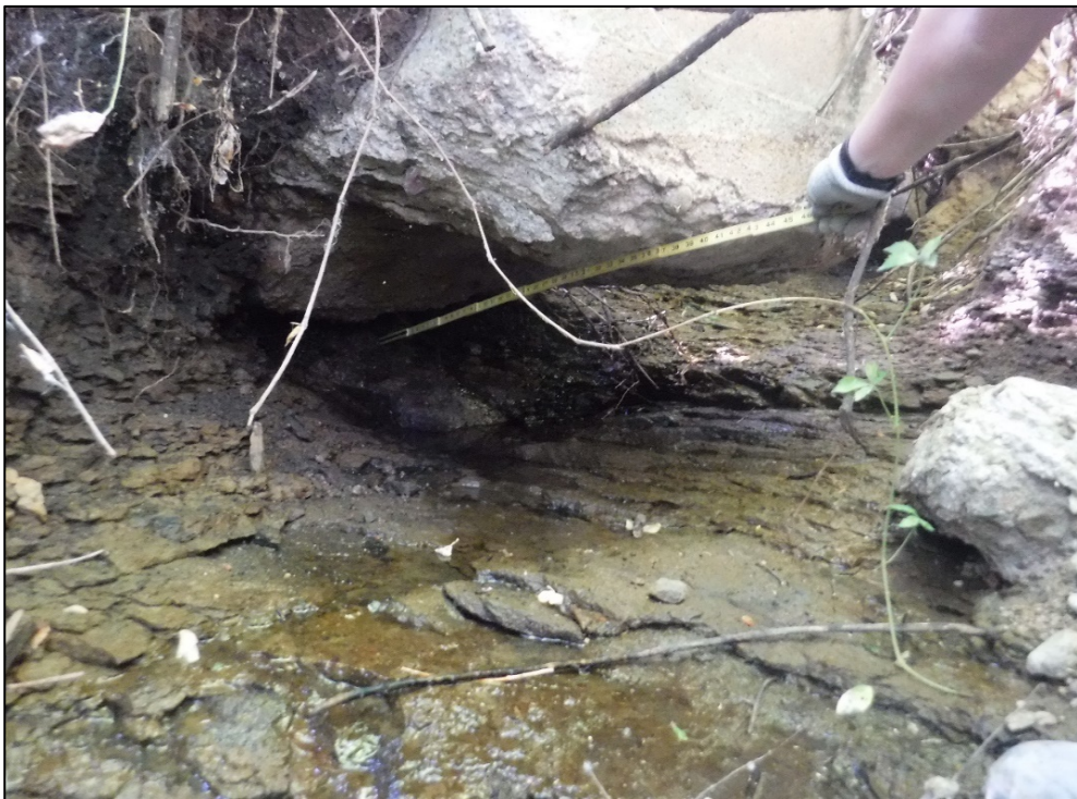
Pier 6 west footing has 10 percent remaining bearing capacity.
