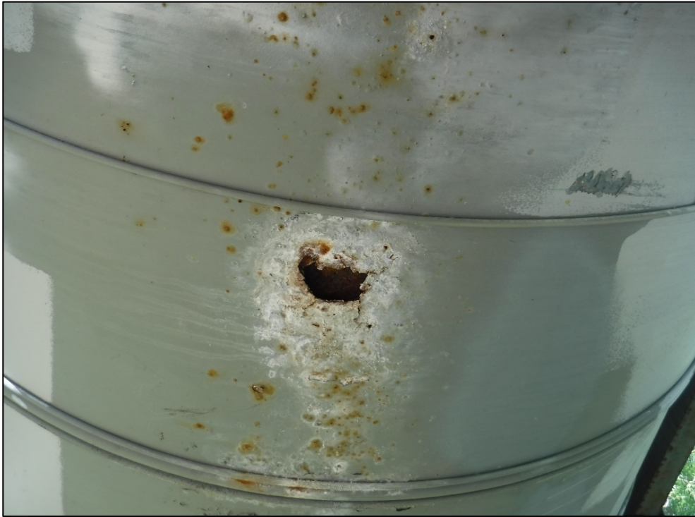
Deck underside in Span 9 has up to 3 inch diameter corrosion holes.
