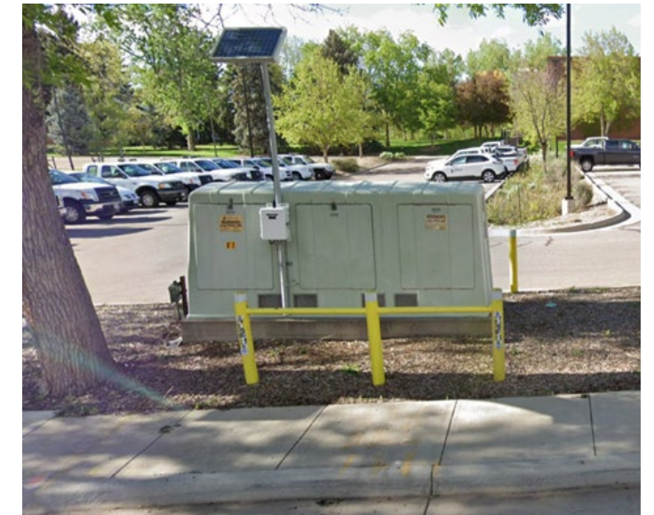
Same XCEL Gas Reg Station viewed from Google Street view
