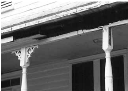
Replace missing original details in kind.
