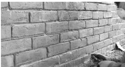
Repoint mortar joints where there is evidence of deterioration.
