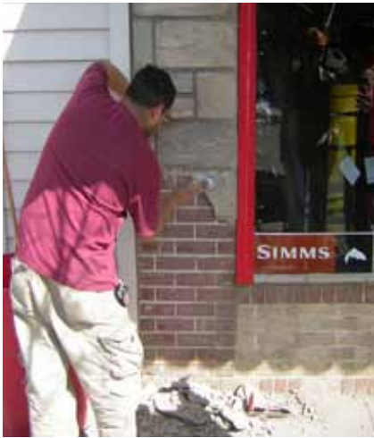
Consider removing later covering materials that have not achieved historic significance. Once the non-historic siding is removed, repair the original, underlying material.
