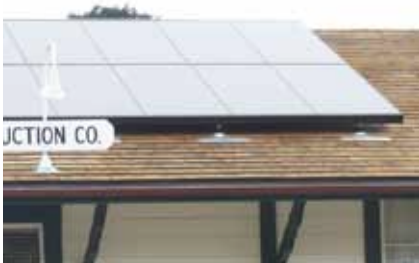
Attach solar collectors to a historic roof in a minimally invasive and reversible manner. In this example the panels are mounted such that the original shingles are saved.
