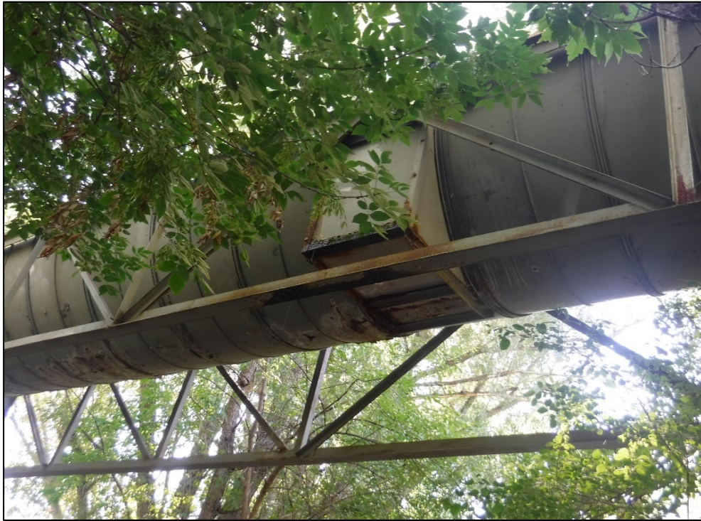
Truss 6A lower chord bent upwards at mid-point looking east.
