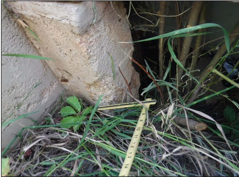
Abutment 14 west end spall.
