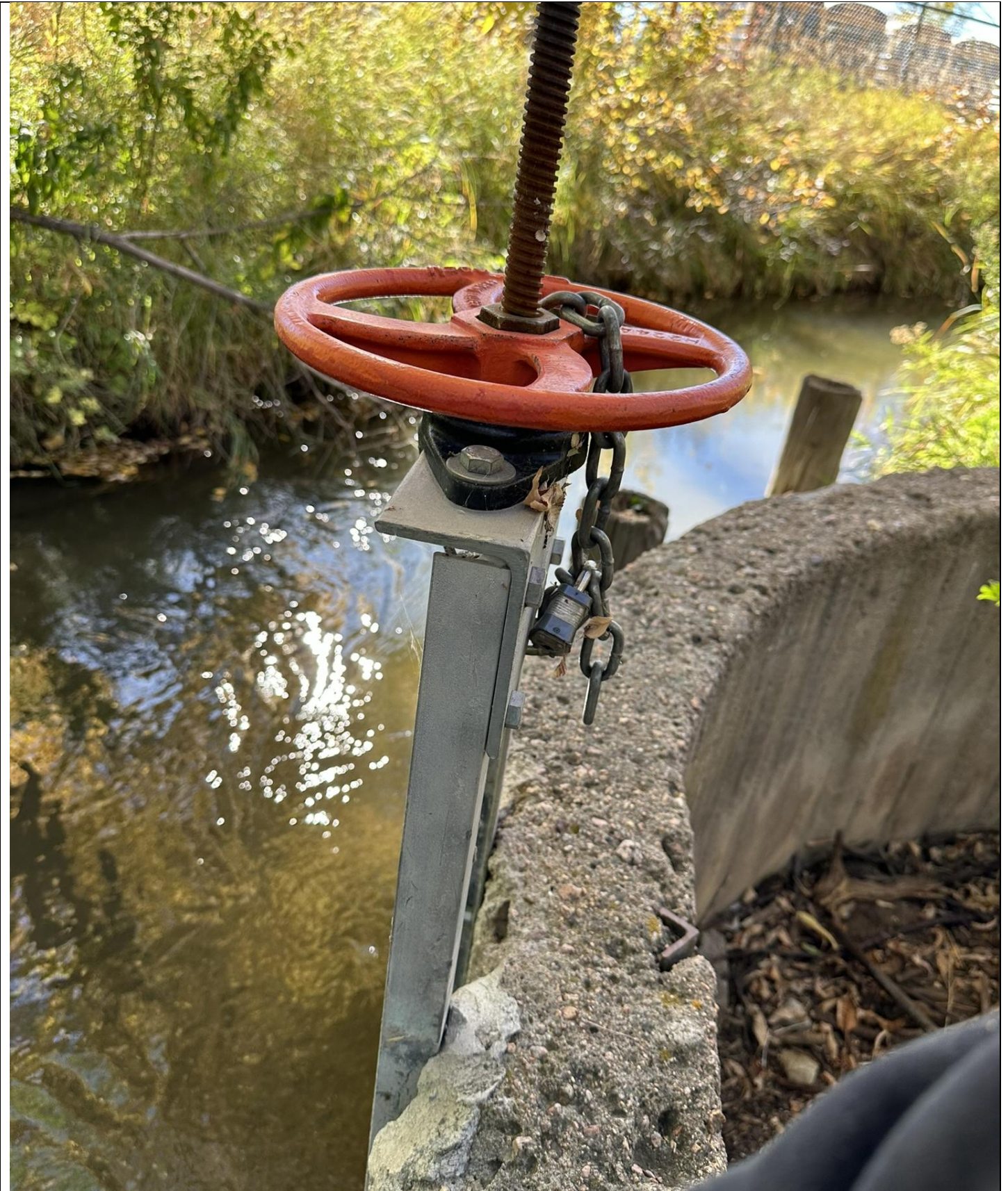
The accessible sluice gate assembly. Negative
