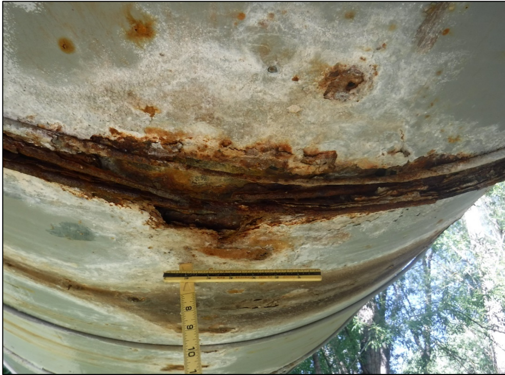
Deck underside in Span 8 along bolt band has R4 corrosion.
