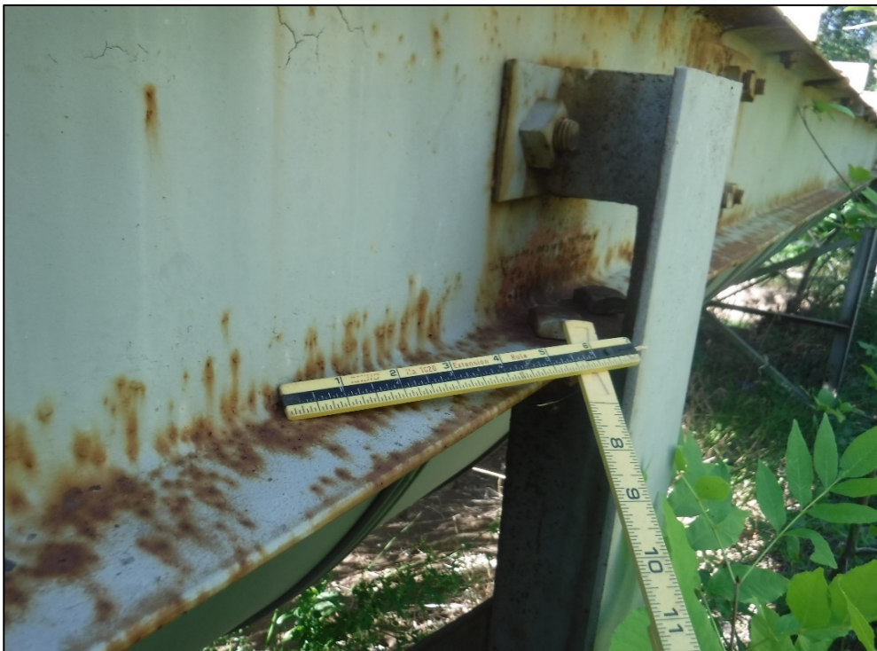
Beam A has R1 corrosion, typical.
