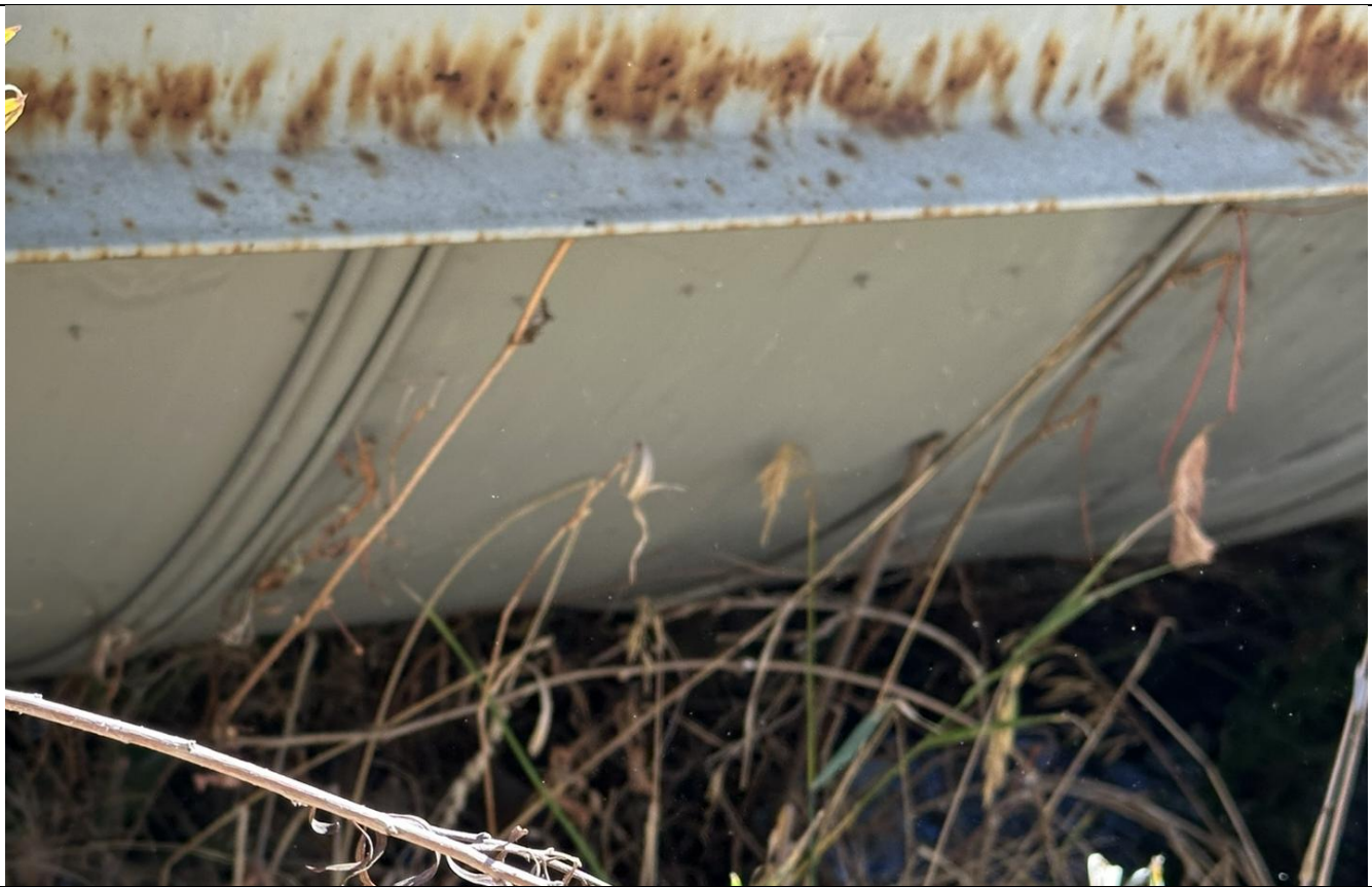
Close-up of the deck. Contains 2.0 -3.1(mg/cm 2 )
