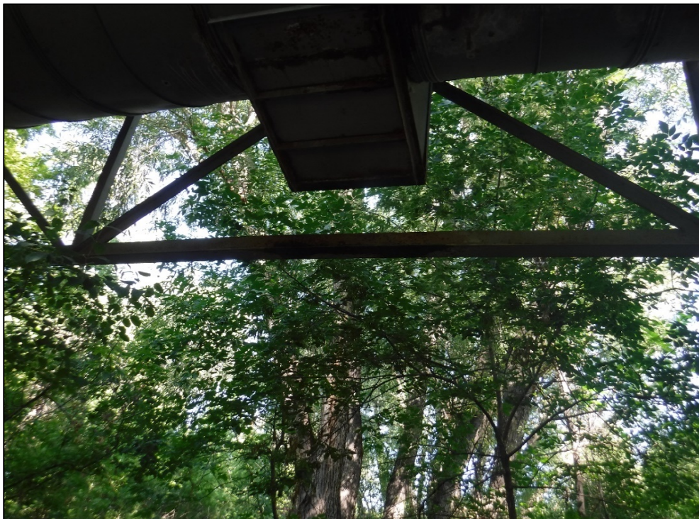
Truss 6A lower chord bent upwards at mid-point looking west.
