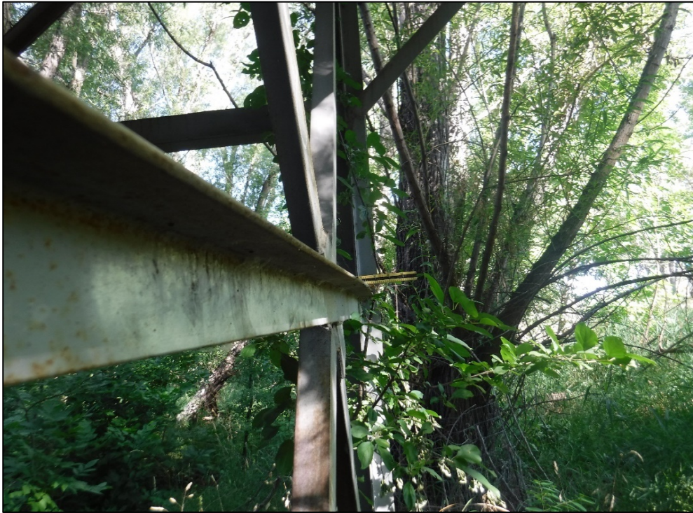
Pier 7 trestle middle horizontal member bent north.
