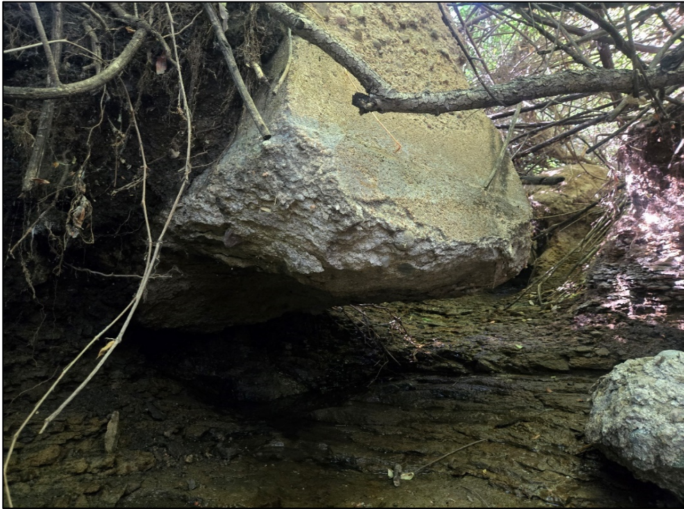
Pier 6 west footing undermined.
