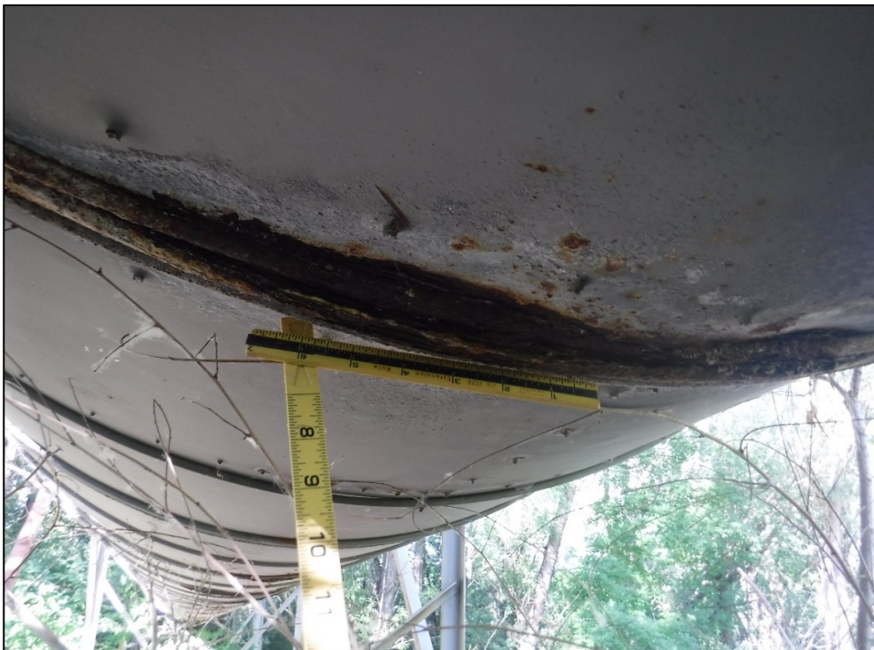
Deck underside at bolt bands has R2-R3 corrosion, typical.
