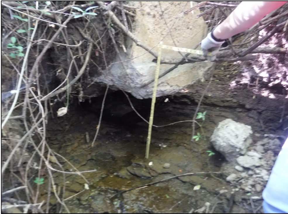
Pier 6 west footing undermined up to 20 inches vertically.
