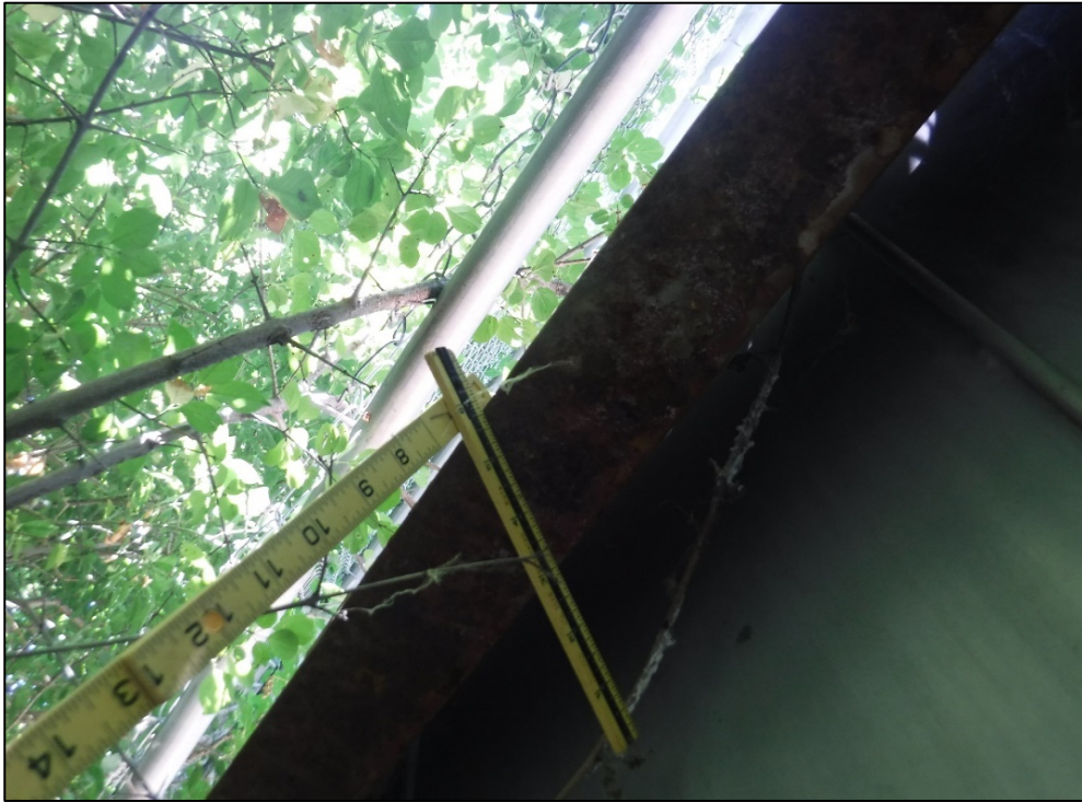
Beam has R1 corrosion, typical.
