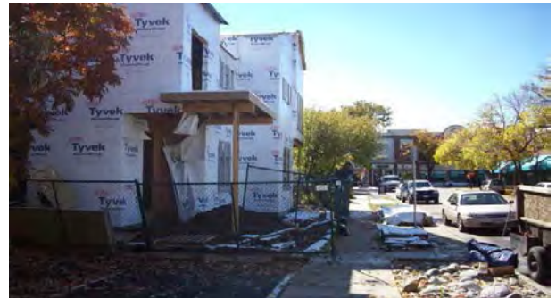
One of several new residences under construction in Downtown Littleton, as of November 2013. This one is a duplex that has replaced a single-family house on South Sycamore Street.
