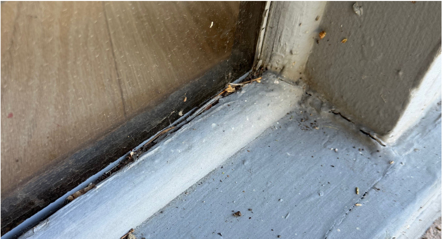
PHOTOS OF ROT DAMAGE TO EXISTING FIXED WINDOW FRAMES
