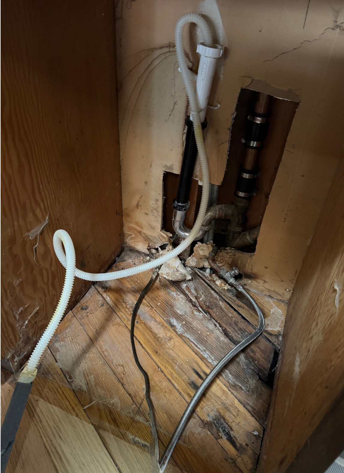
WATER DAMAGE FROM SEWER BLOCKAGE AT DISHWASHER
