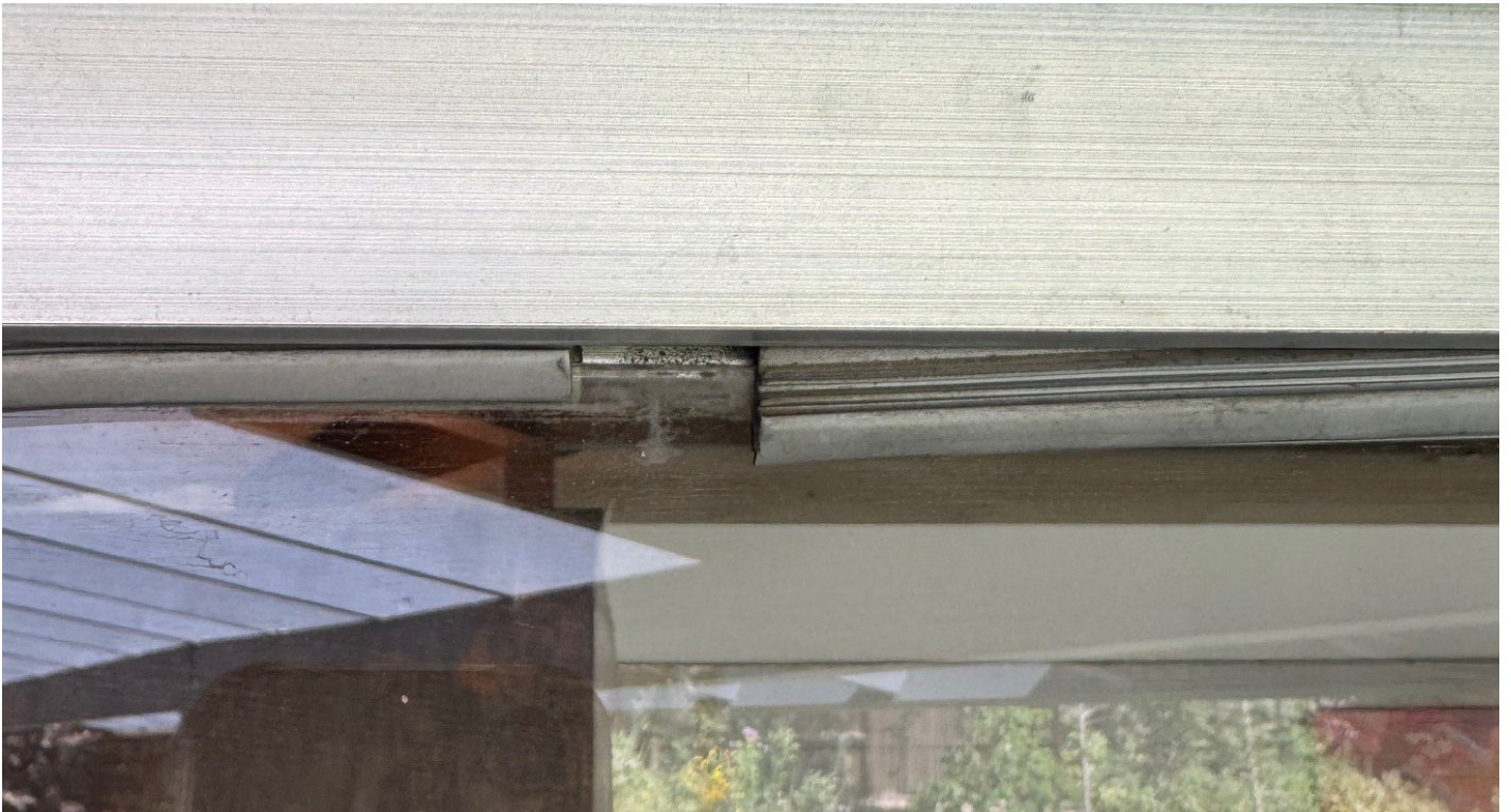
PHOTOS OF DAMAGE TO EXISTING GLAZING STOPS AND WEATHER STRIPPING ON SLIDING DOORS.
