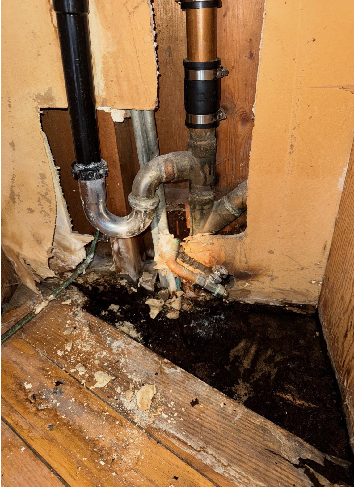
WATER DAMAGE FROM SEWER BLOCKAGE AT DISHWASHER
